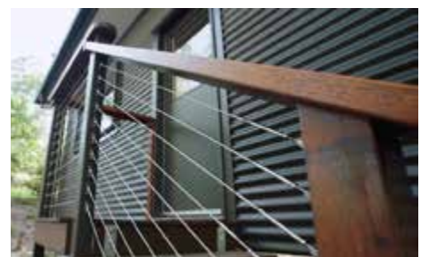
Stainless steel wire with hardwood hand rails to stairs
